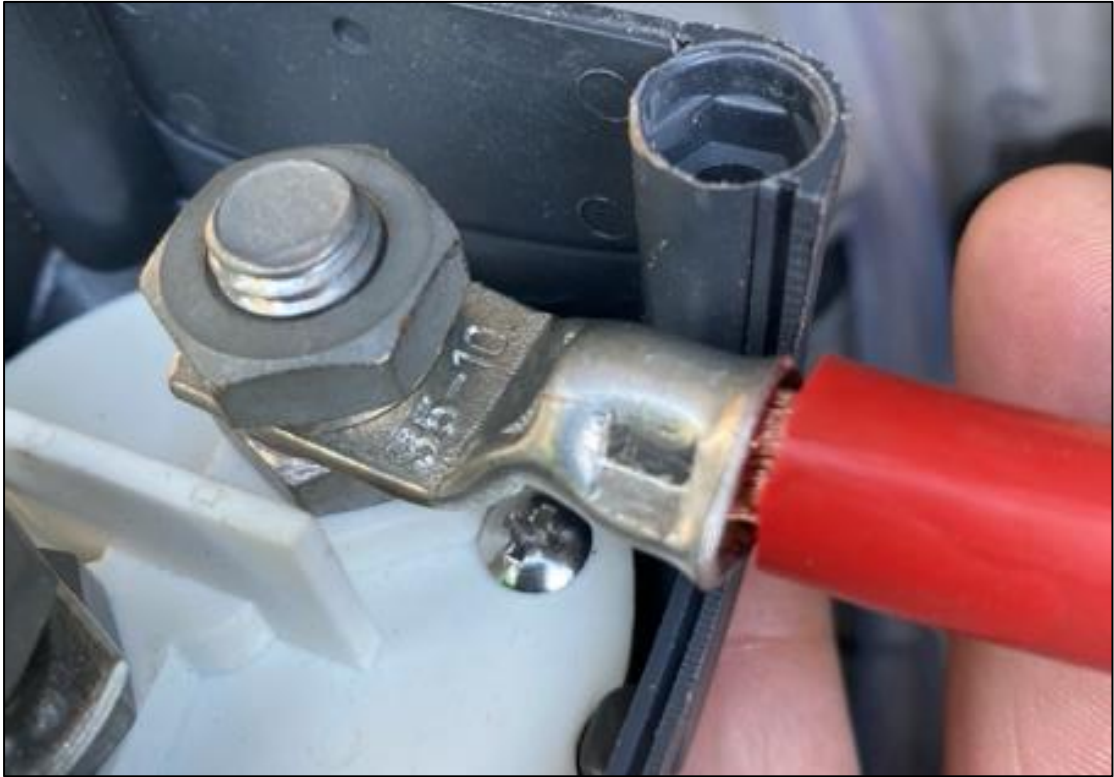
Photograph 5 – Cable end crimped using improper tooling.
