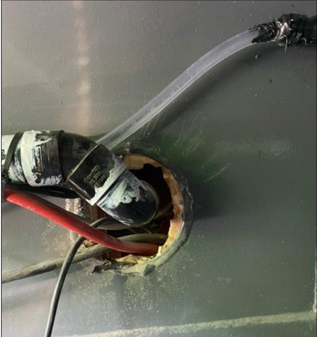
Photograph 10 – Cabling running through bulkhead without chafe protection.
