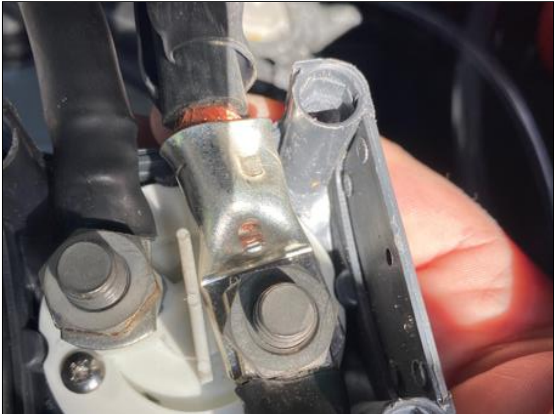
Photograph 6 – Cable end crimped using improper tooling.
