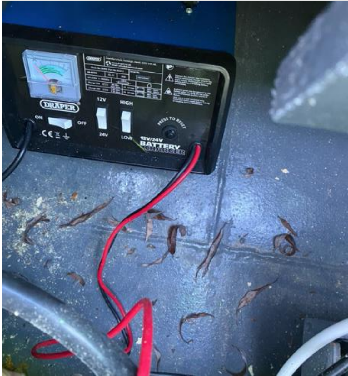
Photograph 11 – Automotive, non-automatic charger connected to bow thruster batteries.
