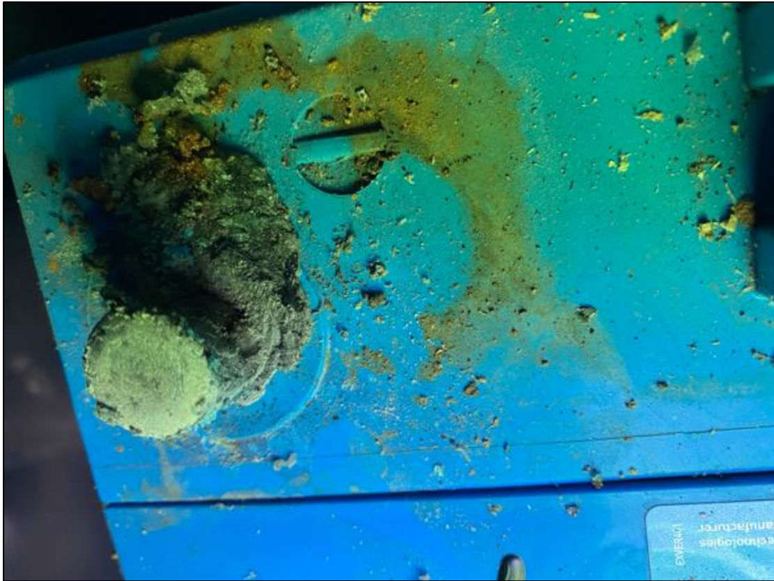
Photograph 15 – Bow thruster battery post (negative) showing severe signs of continuous arcing due to poor connection/loose terminal.
