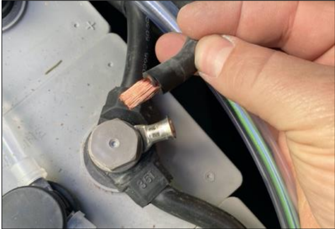
Photograph 8 – Cable end crimped using improper tooling. Pulled out of connection using very light force.
