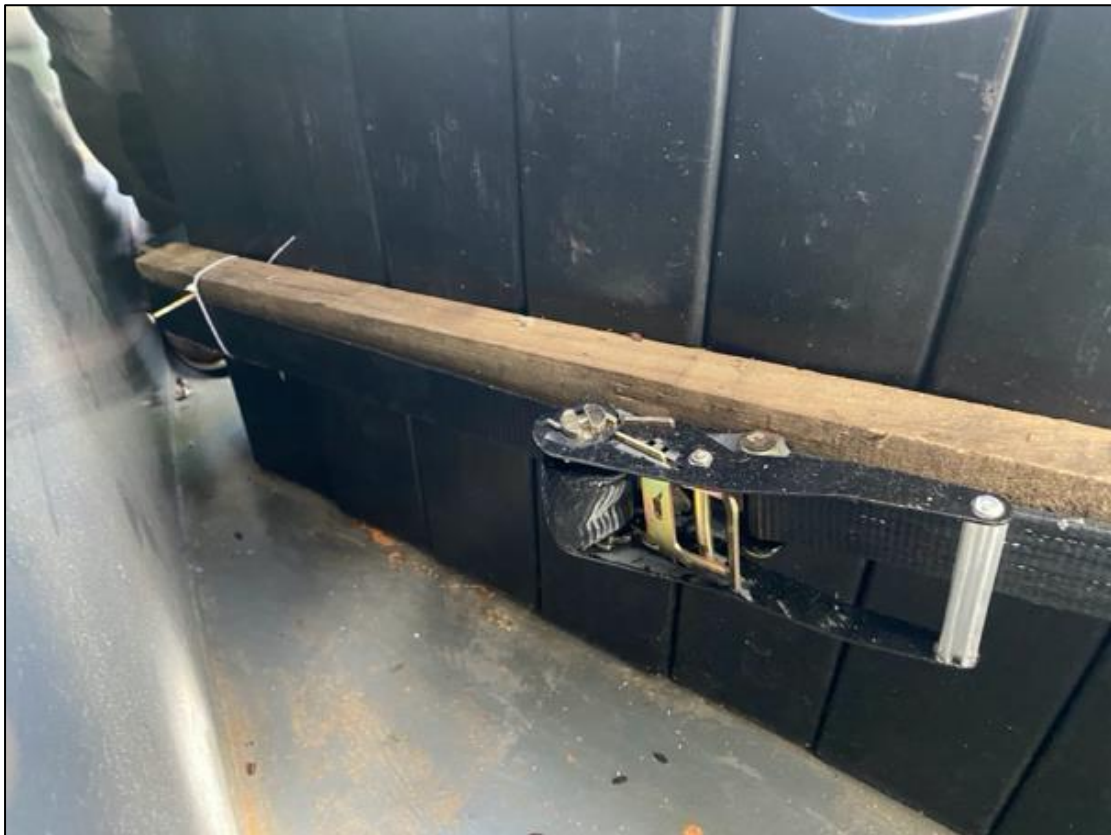
Photograph 4 – Current battery securing arrangement. Batteries installed directly on sole plate.
