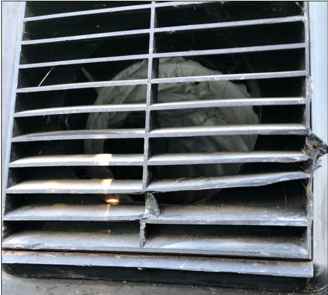
Photograph 18 – Toilet vent/open to hull.
