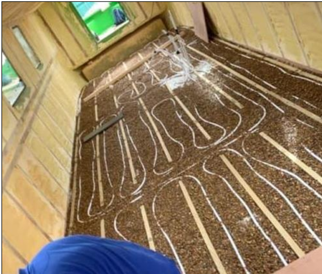
Photograph 17 – Underfloor heating arrangement. Photograph taken during build, taken by owner.
