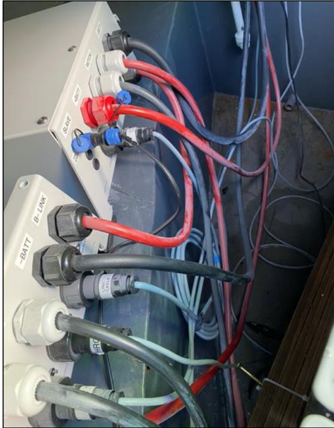
Photograph 3 – Unsupported and unprotected cabling from and to the motor controllers,
