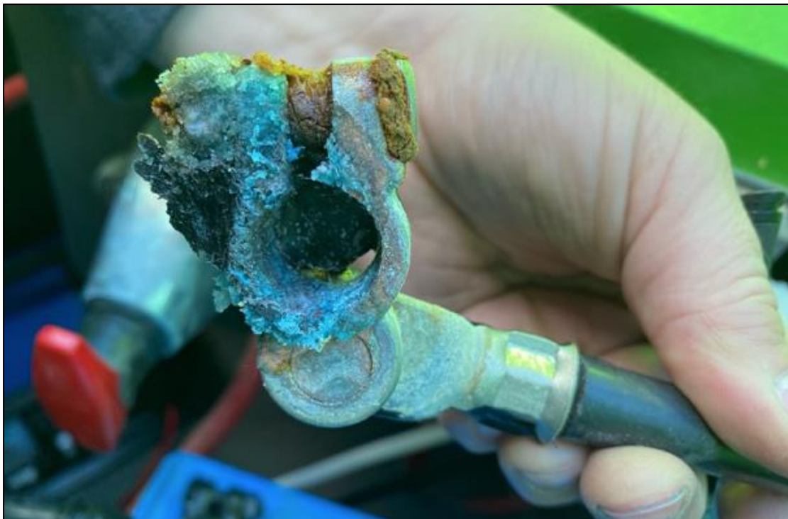
Photograph 14 – Bow thruster battery clamp (negative) showing severe signs of continuous arcing due to poor connection/loose terminal.
