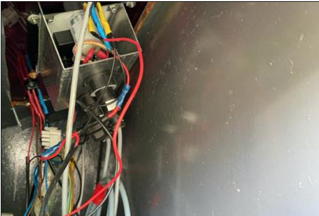
Photograph 2 – Unsupported and unprotected wiring under dashboard.
